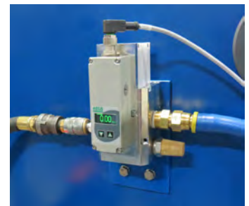
AFPCS Pump Control Mounted to Filter Press
