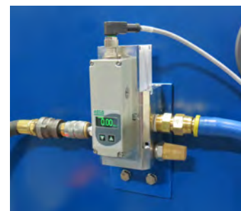
AFPCS Pump Control Mounted to Filter Press
